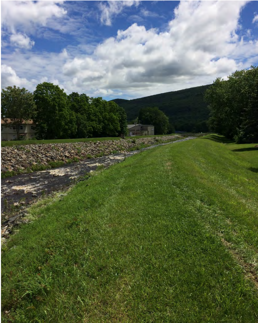
Beer Kill Left and Right Bank Levees Looking East from Just Downstream of Main Street
