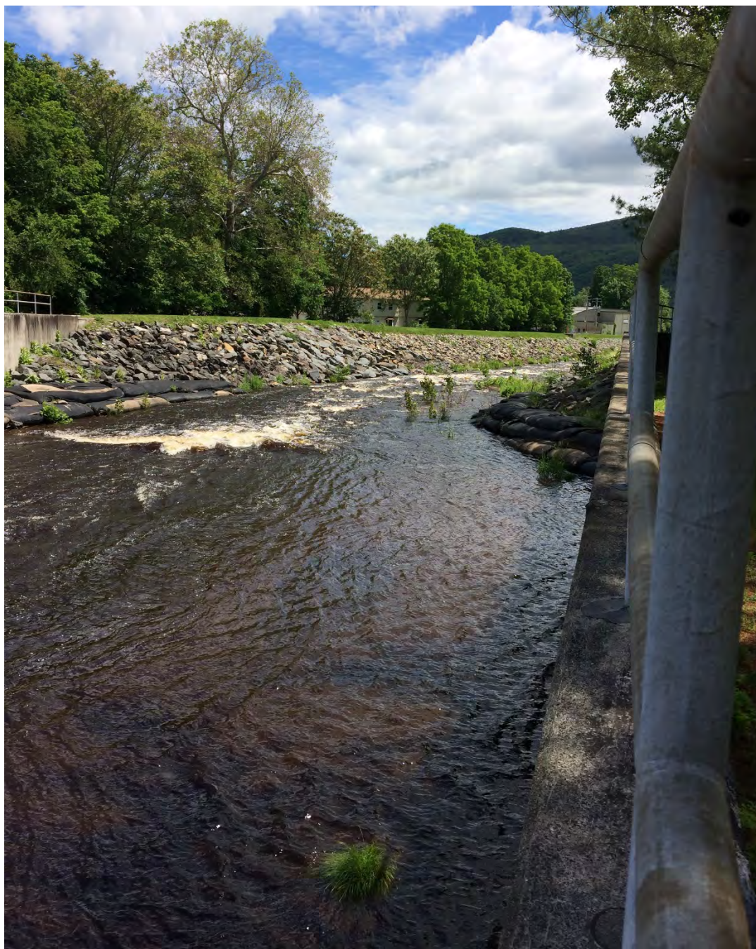
Beer Kill Left and Right Bank Levees Looking East from Main Street
