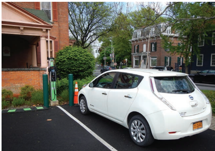
Electric Vehicle Charging Station at the County Office Building Complex
